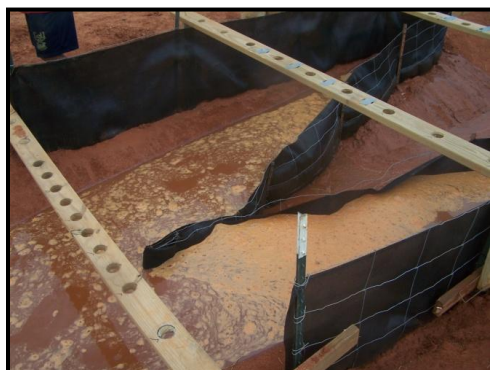
Figure 8. Silt Fence Check Structure
