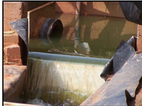
Figure 2. Flow into Channel at Weir
